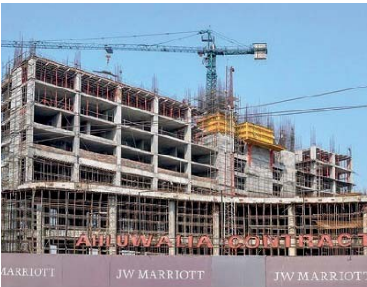
Multi-storey Hotel and Service Apartment with VARIO VT 20 and RCS/VARIO rail climbing formwork systems used for lifting core walls.
