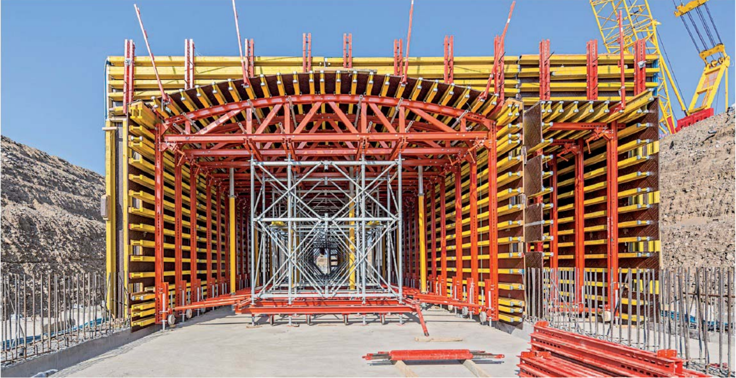
Enabled by PERI tunnel formwork, a rapid four-day cycle per section was achieved at a tunnel construction site near Muscat. Through its cost-effective and flexible design, the side shutter and decking also relied on VARIO VT 20.
