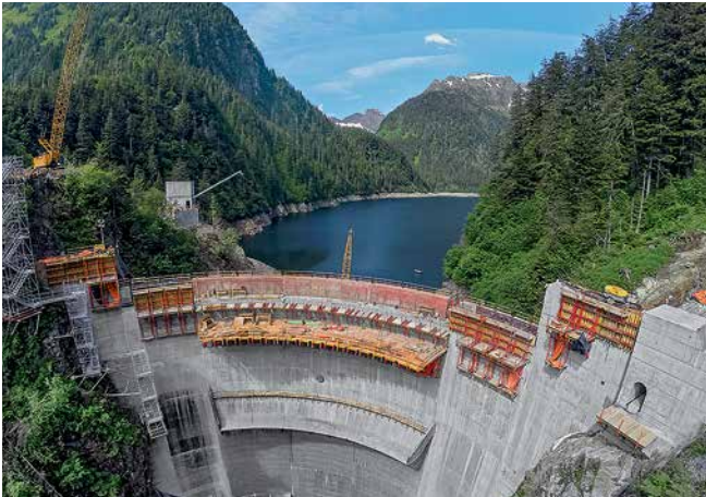
Important dam upgrade project: as part of a hydroelectric power plant expansion in Alaska, the height of the dam wall was to be increased.
