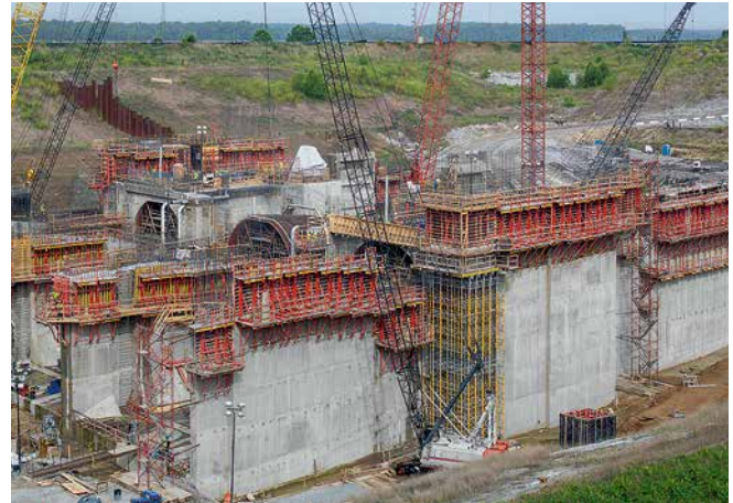
The massive power plant walls were formed in a single-sided process and concreted using the Climbing System SCS.
