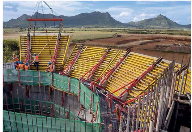
Special suspension points ensured that the formwork elements could easily be lifted into the respective final position with the crane.
