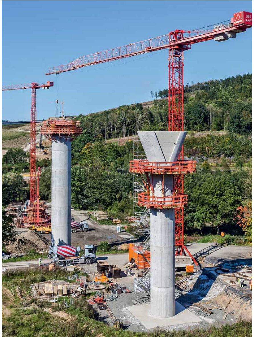
The SCS provided the optimum solution for the heads of these reinforced concrete piers for the composite bridge.
