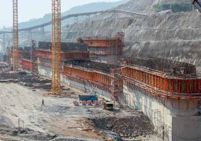
The high flexibility of the Climbing System SCS allowed an easy adaptation to suit all geometries in this dam project.
