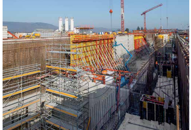
Comprehensive formwork solutions and a high degree of prefabrication also helped to deal with complex building geometries at a depth of 15 m - easily, accurately and on schedule.
