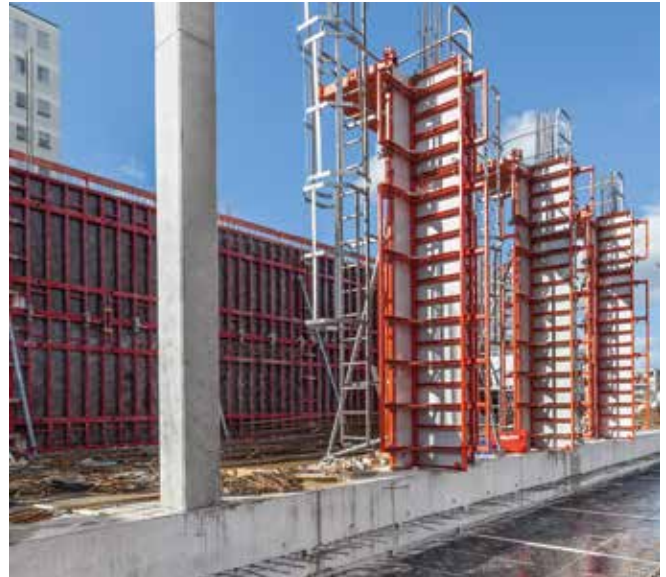
The walls of the "am Hirschgarten" urban district were formed in no time at all using MAXIMO Panel Formwork.
