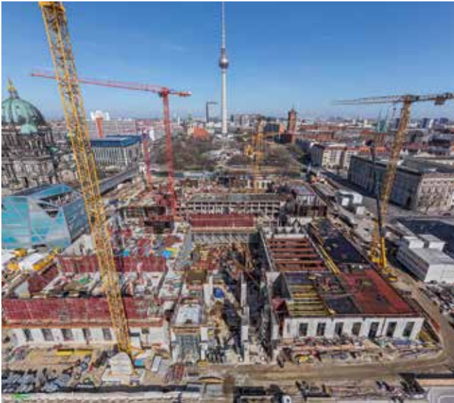
More than 6,000 m 2 of MAXIMO Panel Formwork materials were in simultaneous use during construction of Berlin's City Palace.
