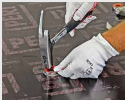
... to MX 18. This allows for a quick and easy on-site exchange process at your construction site.
